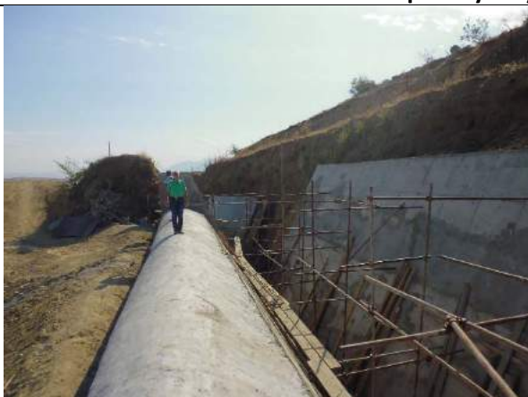
Reparation weir crest. Poor concrete. Narrow spillway canal
