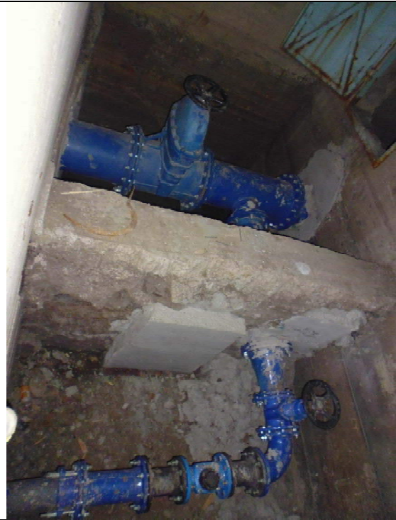
Irrigation outlet valves
