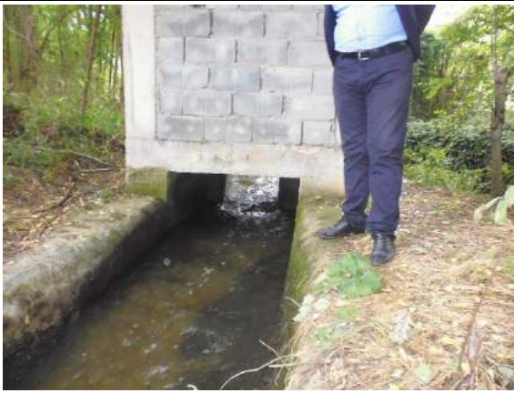
Measuring flume not working
